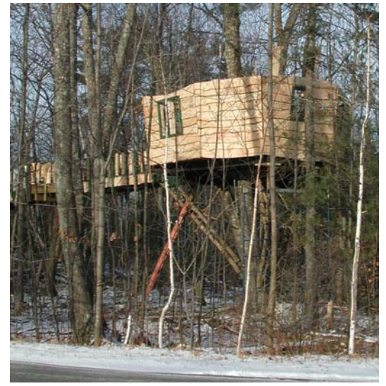
Construction of the treehouse continues to defy gravity as walls, roof and cupola near completion.
